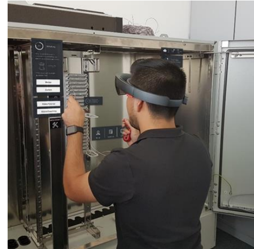
Wiring in a street cabinet
